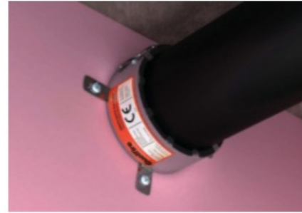
Fire collar fitted to wall
