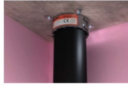
Fire collar fitted to ceiling/floor
